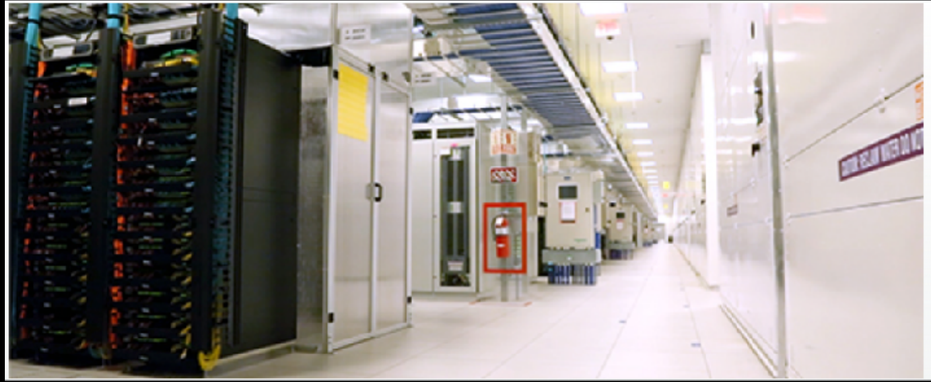
Amazon web services data center Courtesy amazon.com
