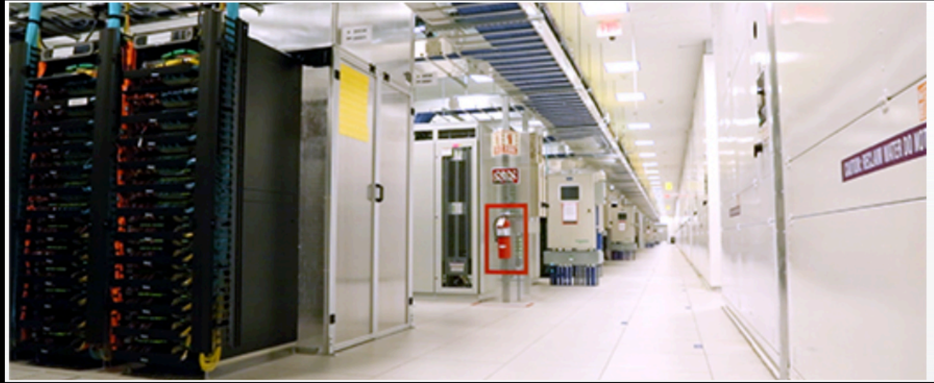
Amazon web services data center Courtesy amazon.com
